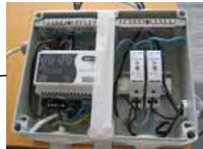
Blind control unit
