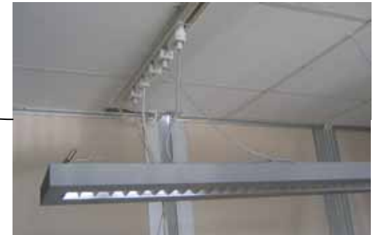
Luminaires with Dali-ballasts
